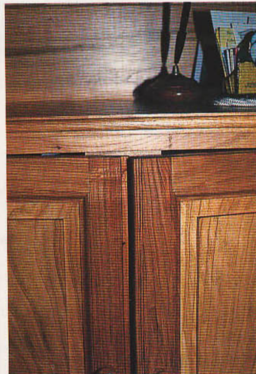
The rebates on the meeting stiles should be cut after the doors have been hung
